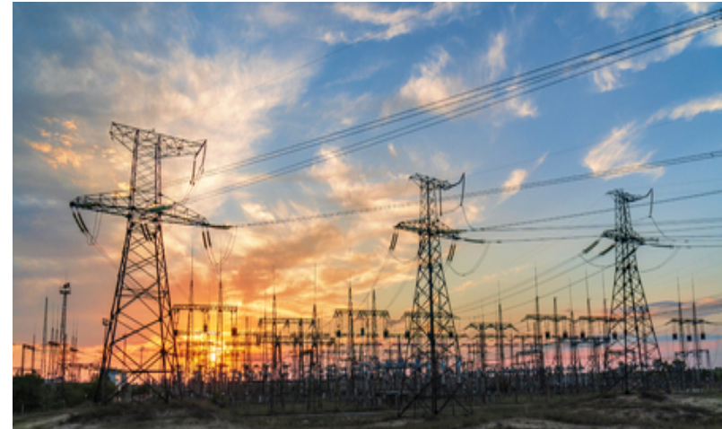
Figure: Electrical systems
